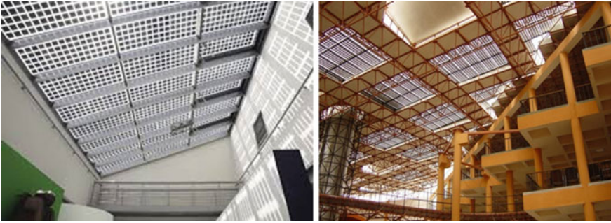
Fig. 2.9 View of roof-integrated semitransparent photovoltaic (PV) module
